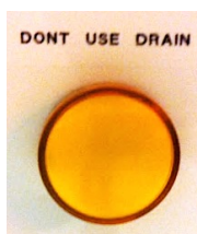
Figure 4: Warning light for neutralizer.
