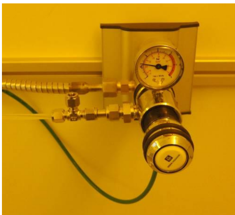
Figure 5: N2 pressure regulator for e-Line vacuum chamber vent.
