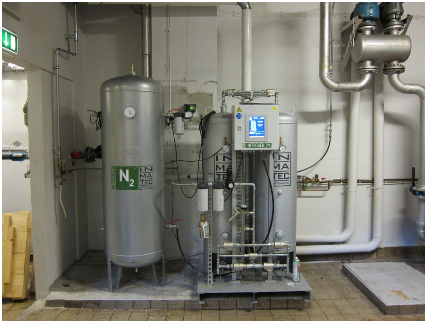
Figure 12: Nitrogen Generator located in Fyrrum (142)
