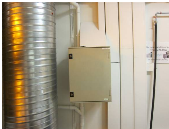
Figure 8: Box with processor regulating the inlet air and what is extracted via fume hoods located in room 268.
