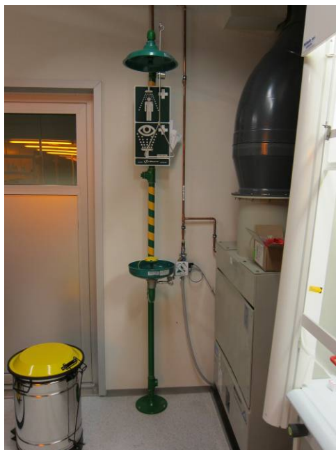
Figure 31: Emergency shower and eye wash.
