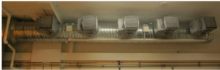
Figure 7: Air inlets with 5 on/off shutters in room 268.
