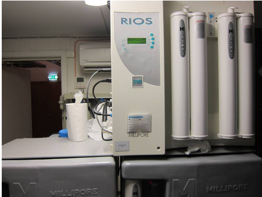
Figure 19: Millipore Di-water unit with storage tanks. Check display for maintenance messages!
