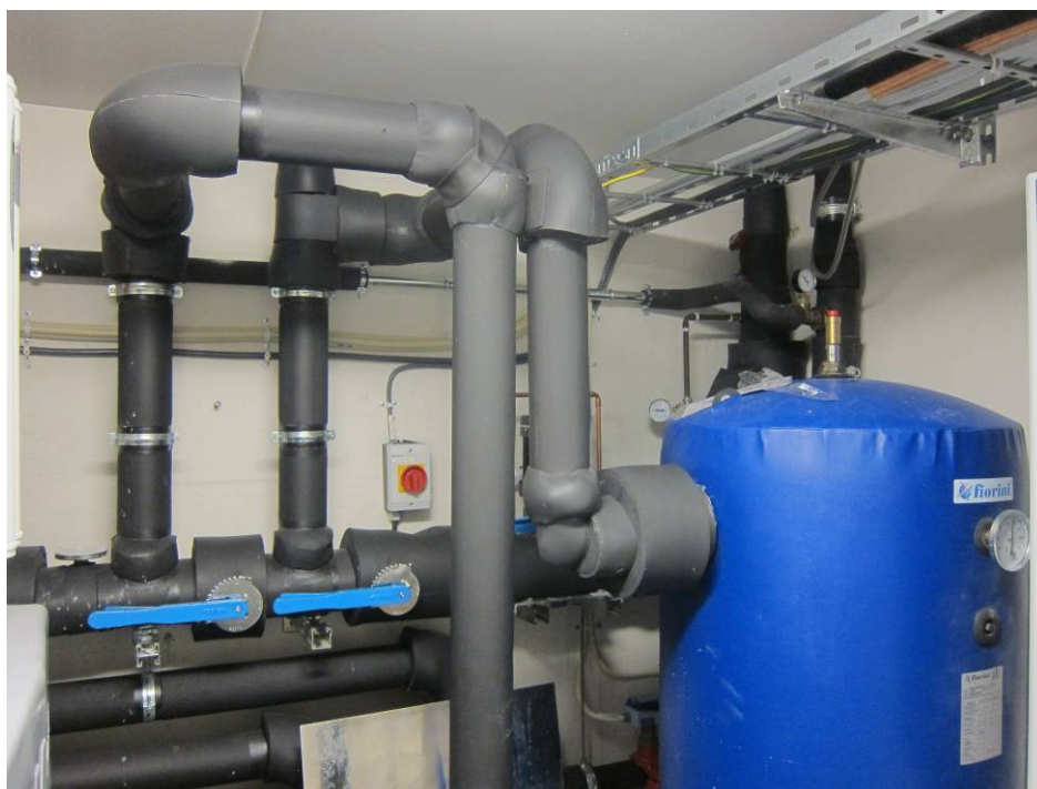
Figure 2: Piping in room 168 of cold water installation, including buffer tank.
