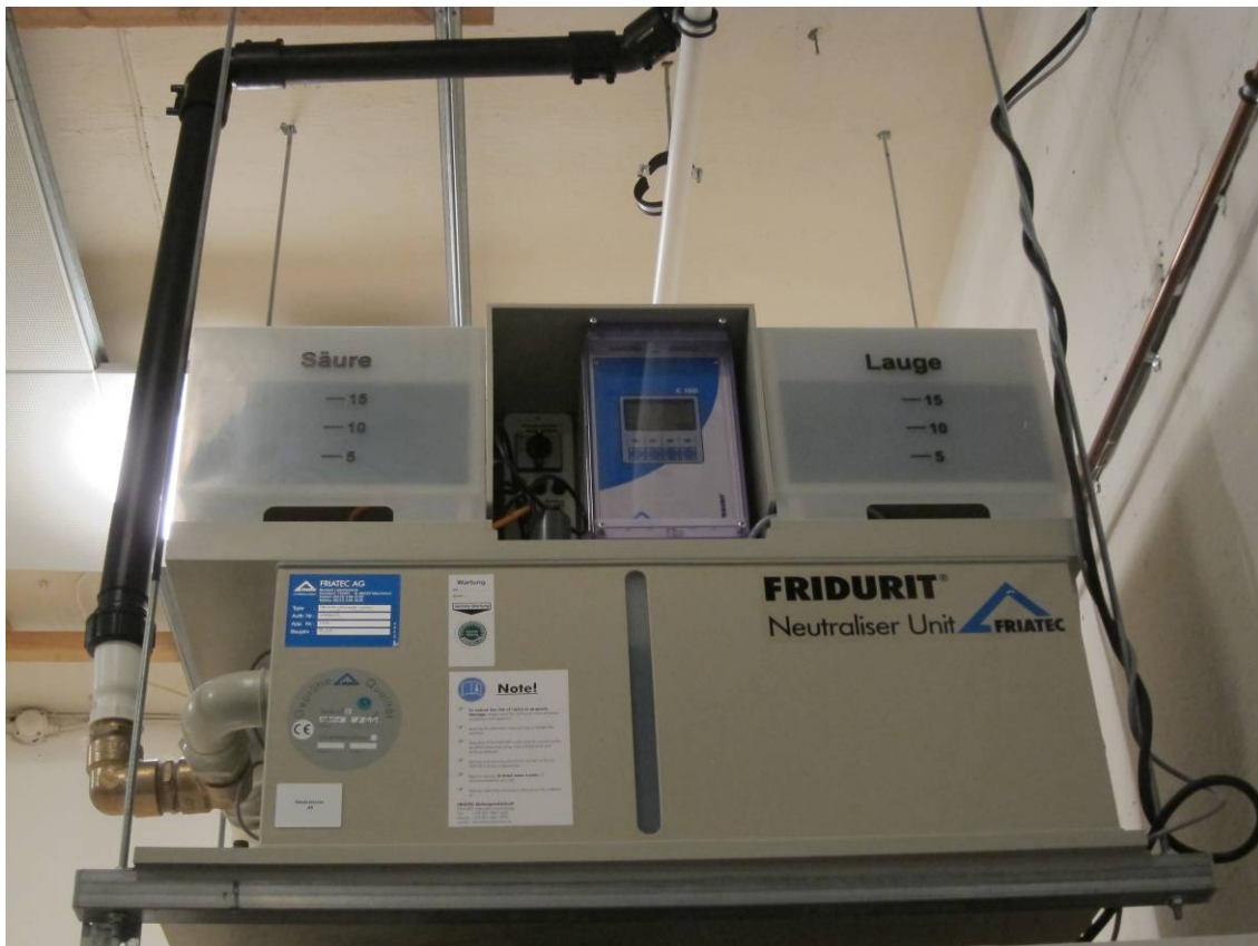
Figure 22: Fridurit Neutralizer unit located in room 168.
