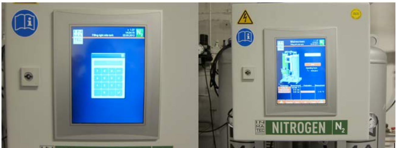
Figure 13: Touchpanel log-on screen and Parameters monitor. The purity should show 100% during normal operation.
