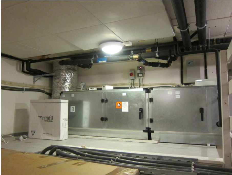
Figure 6: Fresh air supply tunnel with heating, filtration, fan and air conditioning stored in room 168.
