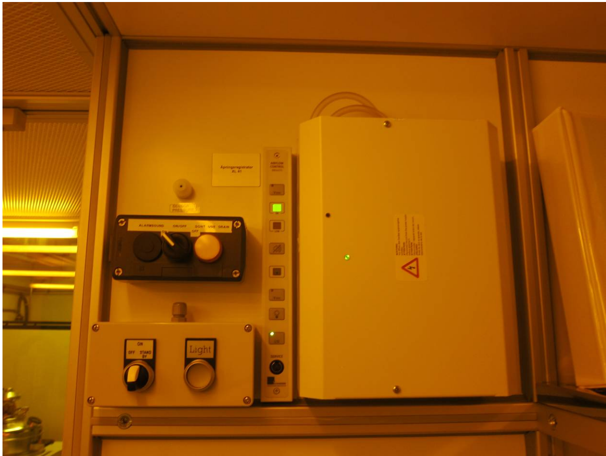
Figure 28: Fume hood controls.
