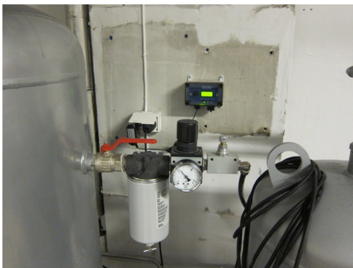
Figure 16: Oxygen deficiency monitor in Fyrrom next to Nitrogen Generator. The output pressure regulator of the Nitrogen generator can be seen in the front
