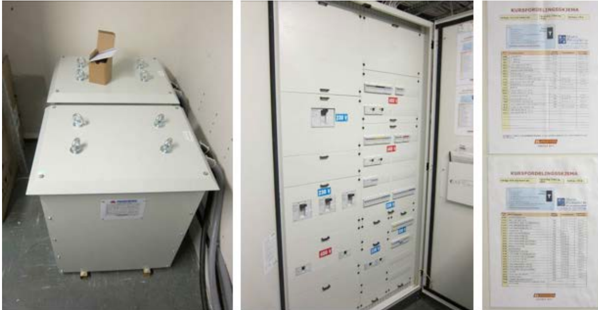
Figure 1: Transformers for 400V 3-phase and power distribution panel in room 168, with documentation
