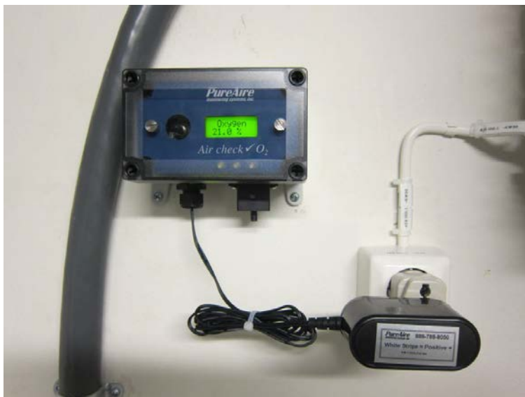
Figure 15: Oxygen deficiency monitor. Check operation by spraying for example helium or nitrogen from a bottle at the sensor located underneath the box.
