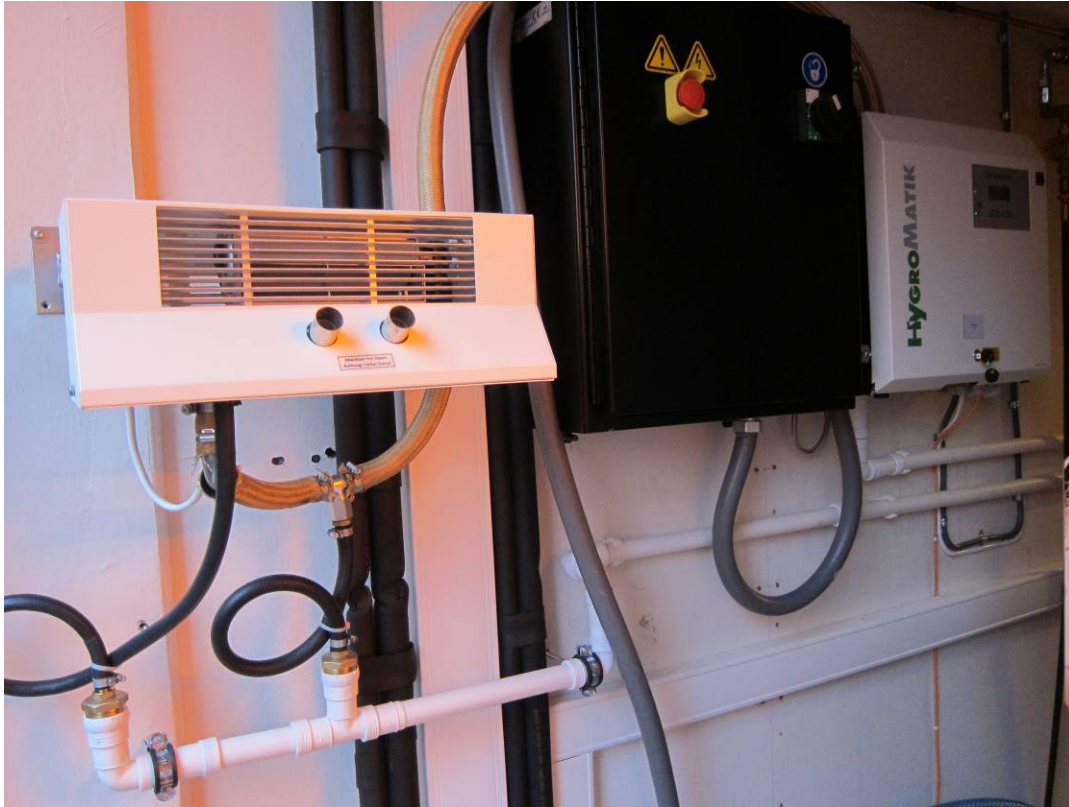
Figure 30: Hygromatik steam humidifier. Outlet is on the left and control box on the right. The black box in the middle is the Power distribution box for the Plasmatherm.
