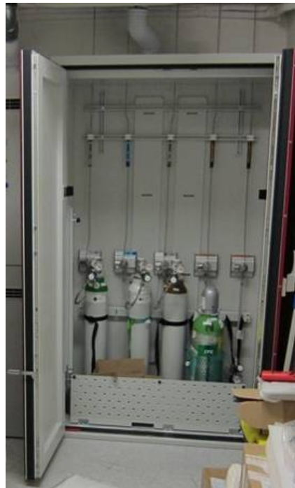
Figure 17: Storage cabinet for the Process gases used by the RIE (Oxygen, Helium, Argon, CHF 3 , CF 4 )
