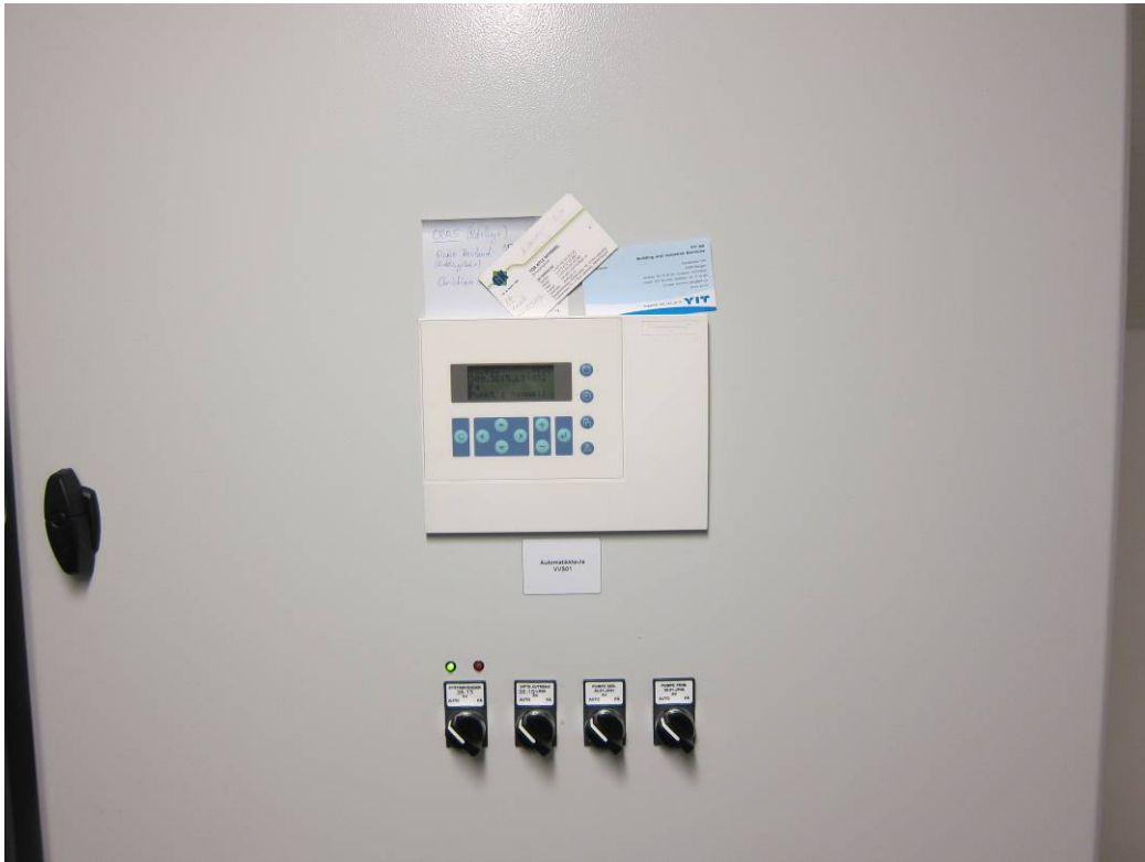
Figure 9: Control box for cold-water supply and ventilation system.
