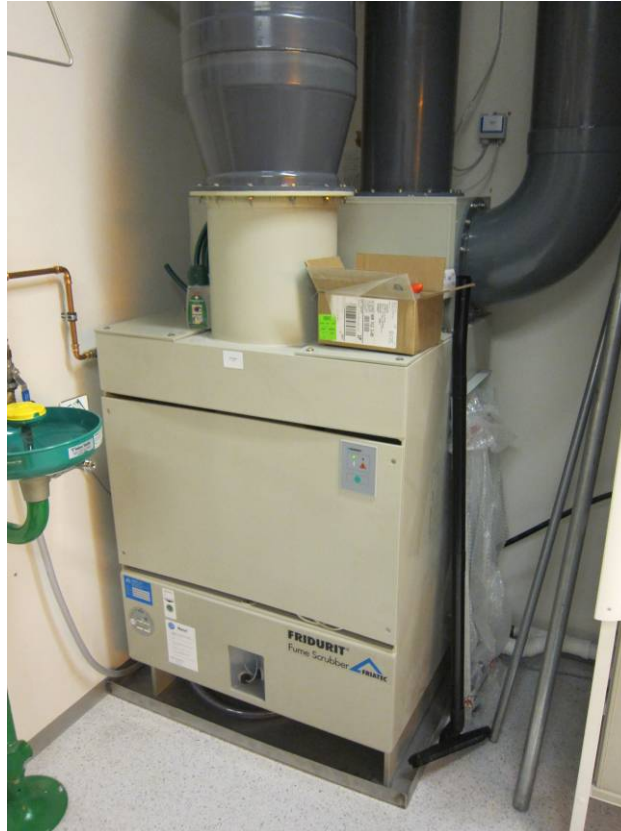
Figure 23: Fridurit Fume Scrubber located in room 268. Call Firatec directly for service.
