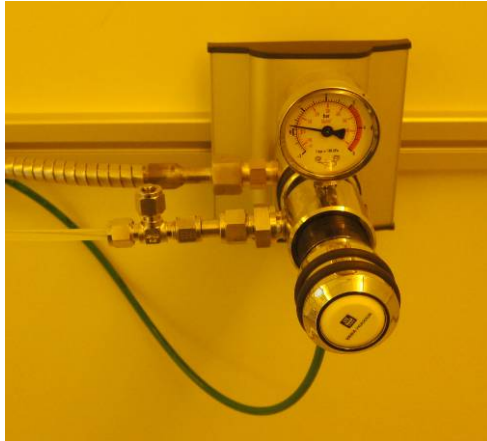
Figure 6: N 2 pressure regulator for e-Line vacuum chamber vent.
